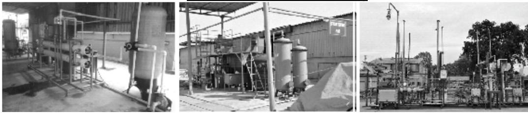
DM Water Plant
